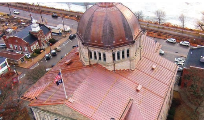
Top to bottom: Lady Liberty undergoes repairs; sheet metal mechanics custom-fabricated new copper flashings, gutters, downspouts and ventilation pieces; an aerial view of Bradford County Courthouse's new roof systems
